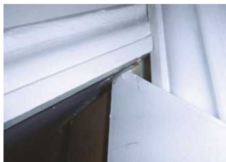
24 Detail trimmed to allow door to open
