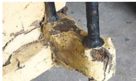
So badly affected it's friable
