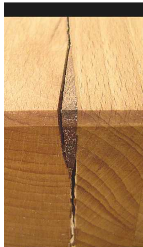
Splits that have opened out
