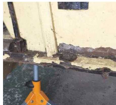
Joints rotted out
