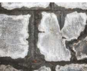
PIC 9. ... and drying: tackling the rainwater problem has meant the cellar floor has begun to dry
