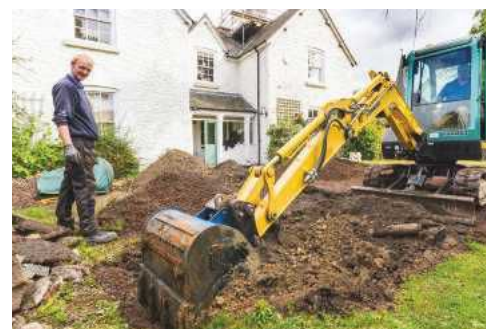
PIC 7. The root of the problem: addressing the causes of damp may mean serious digging...
