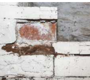
PIC 8. Wet: the timber edging on the steps down to the cellar have rotted, thanks to extreme damp
