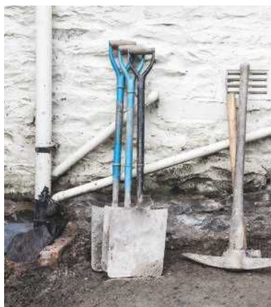
PIC 6. Tired drains, raised ground levels, and blocked-off air vents have all contributed to damp at The Old Vic'
