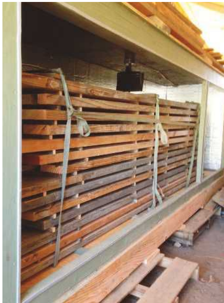
A dehumidifying kiln
