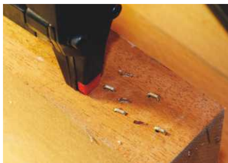
Initial fixings were left proud and required adjustment of the outlet pressure
