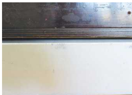
PIC 1 (a). Plywood on original board, which was still OK after some 80+ years
