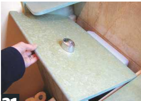
31 This panel lifts out to give access to the cistern and pipework. A small shaped panel is fitted next to the sink
