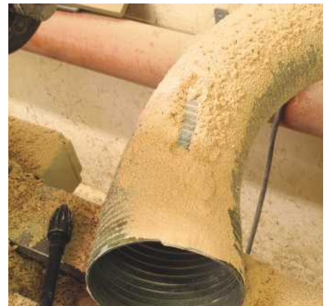
▲ Pic.24 You can see the amount of dust this will create. The 4in pipe cannot cope with these quantities so, as I mentioned earlier, please protect yourself from the dust
