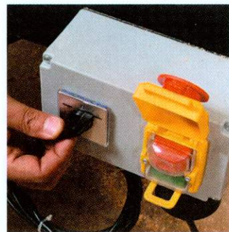
For safety you need to select the function on the NVR switch box
