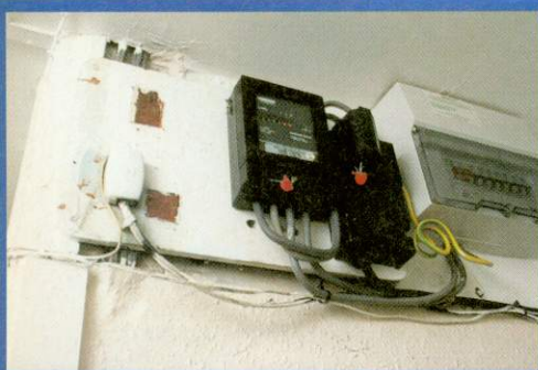
Before: an ugly mess of cables and meters just inside the front door. Mmmm.... lovely
