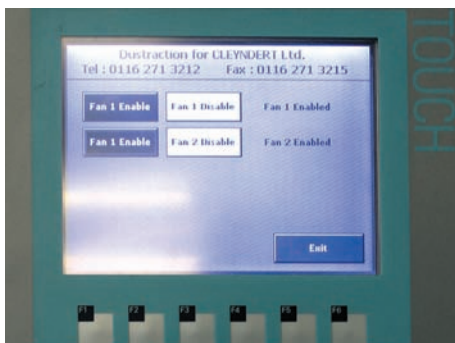
Below. Control made simple with a fully sequenced touch-screen HMI panel.
