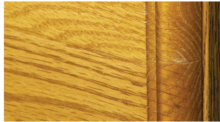
Why is the crack at the joint?
