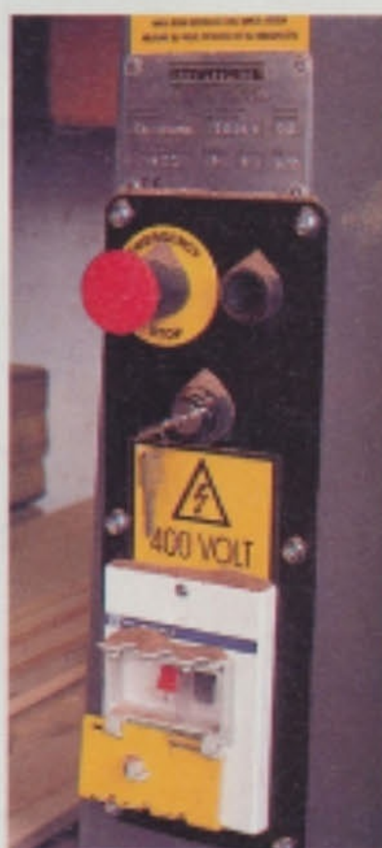
The switch gear, which we found confusing!
