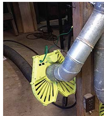
Green retrofit. GrnGate's blast gates can be installed in any dust-collection system. The gates automatically open and close when you turn machines on or off.
