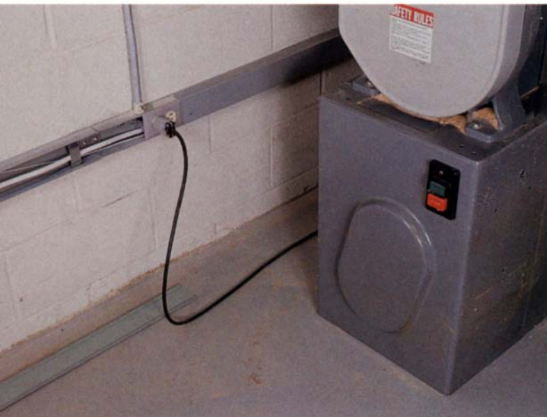
A raceway is a practical way to run new outlets along a concrete wall. By removing the metal cover, as shown here, new circuits can be wired and outlets moved or added at any time.
