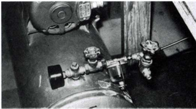
New valve/fitting arrangement controls vacuum to press.
