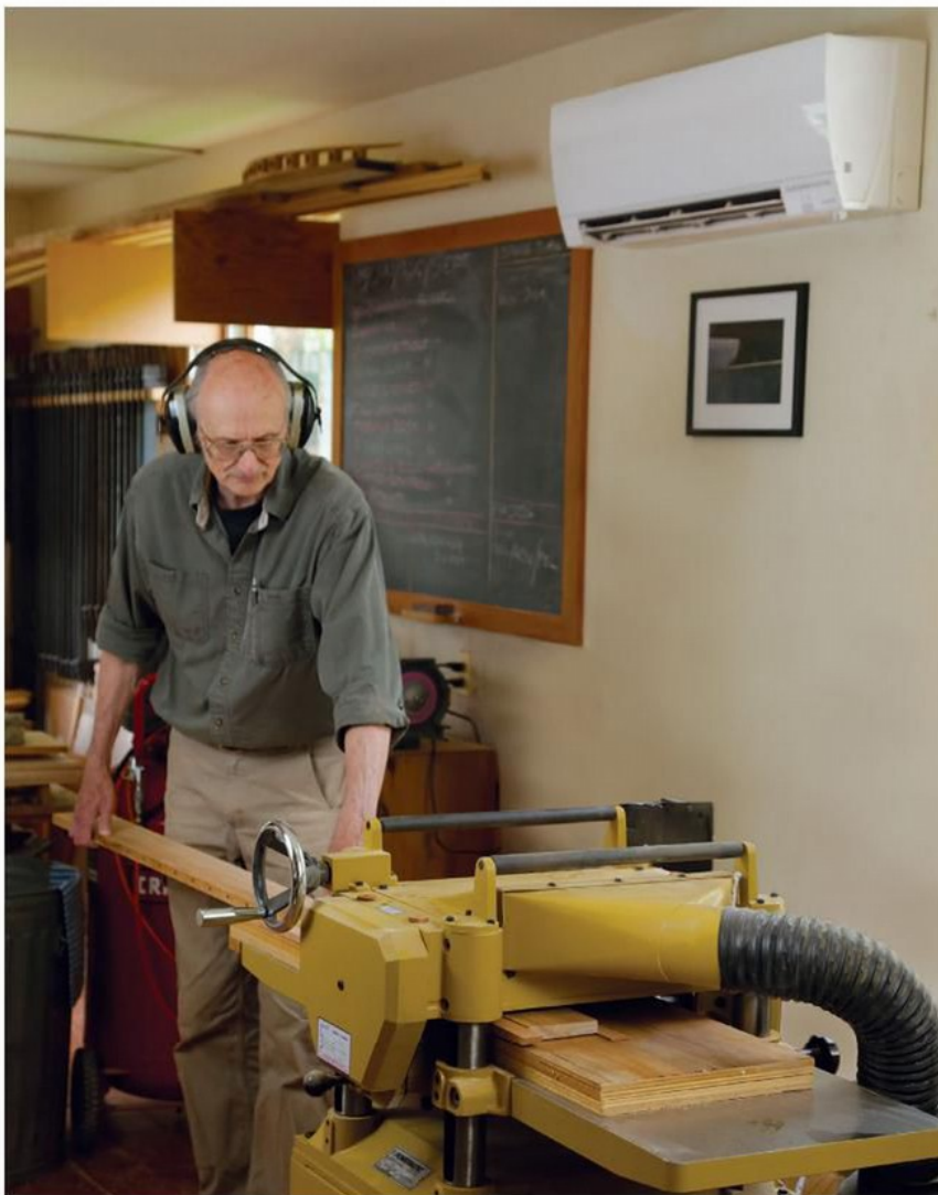
Up and away. Wall-mounted mini-splits, like this one in contributing editor Christian Becksvoort's shop, go high on the wall, so they don't take up valuable shop space.
