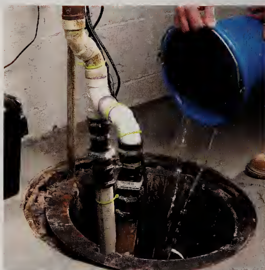
Test your sump pump: Dump water down the sump pit to raise the water level, and make sure the pump is ejecting the water properly.
