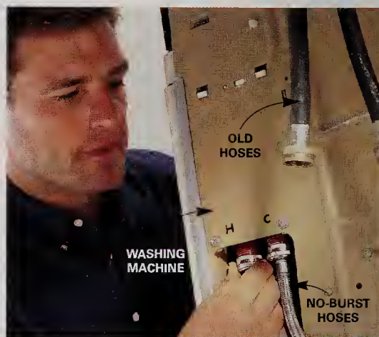
Stainless steel braided (no-burst) hoses last longer than rubber or plastic hoses and are less likely to leak. They also prevent mice from gnawing through the lines.
