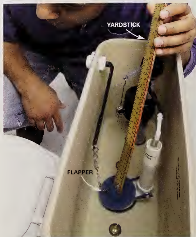
1 PUSH down on the flapper with a yardstick and listen. If the sound of running water stops, the flapper needs replacing.
