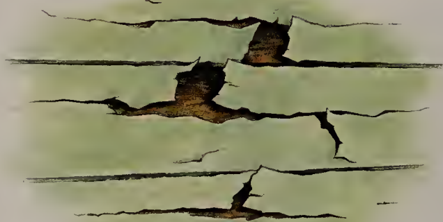
Fig. B: Excess moisture getting behind the siding
