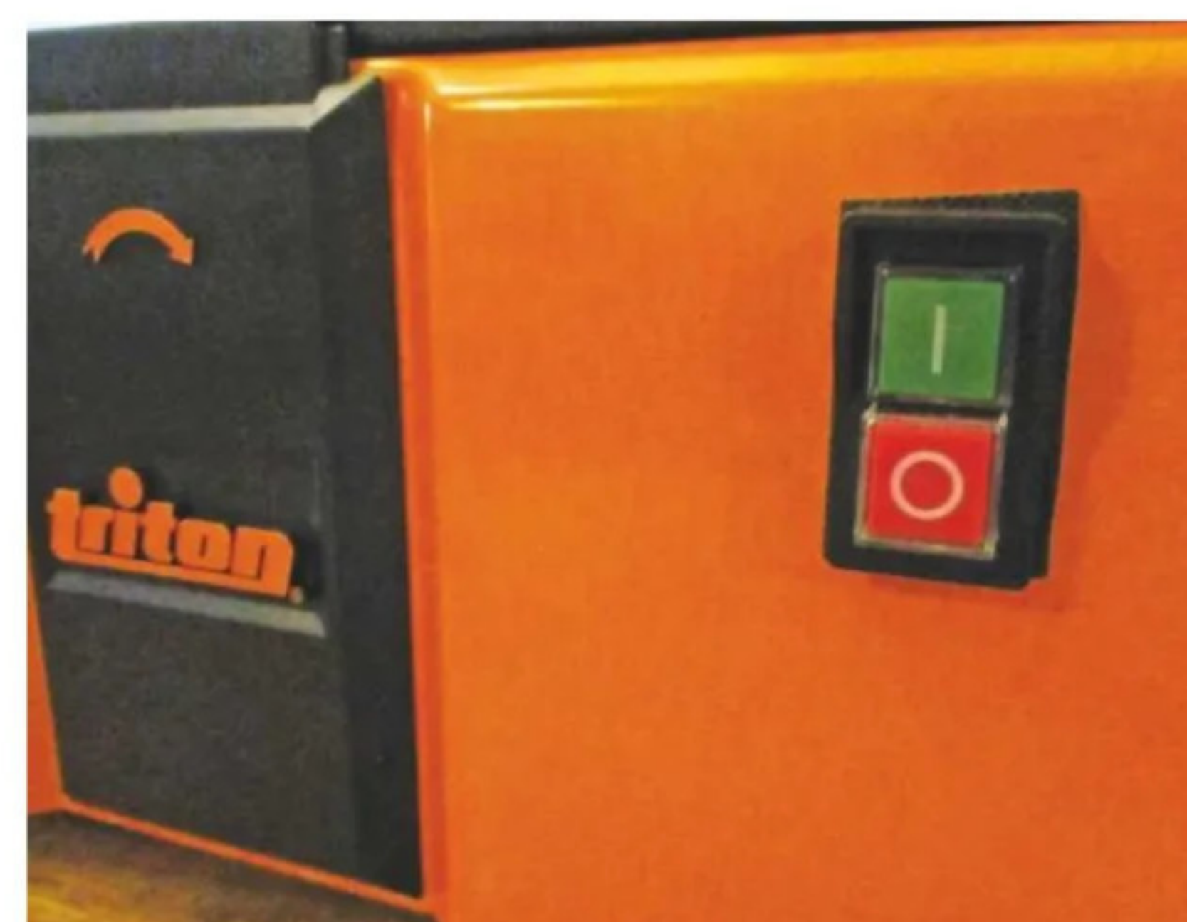
Well placed no volt switch and direction of rotation clearly shown
