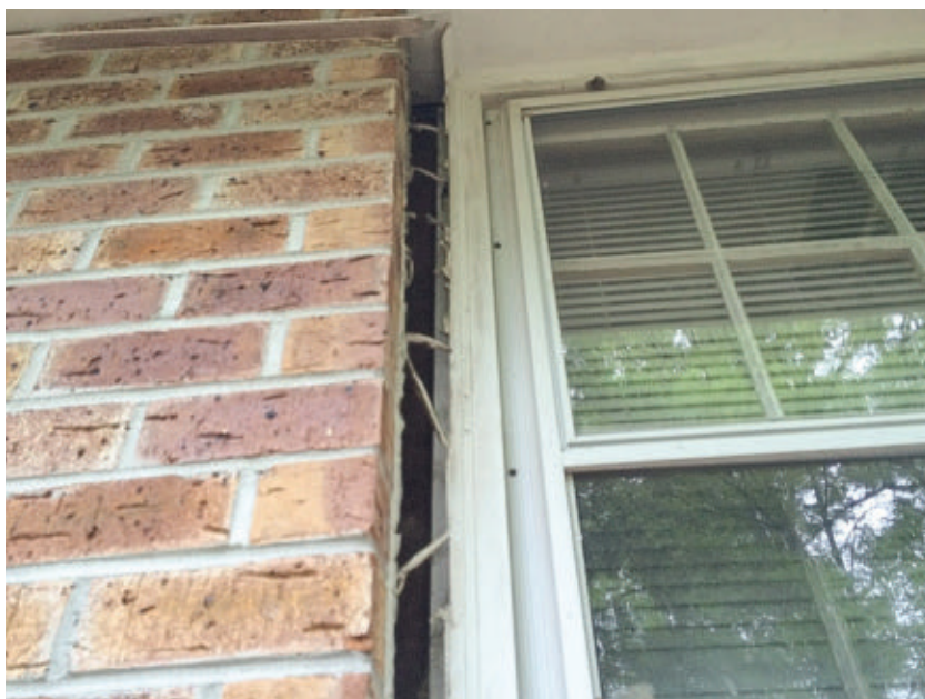
A gap around window frames can be signs of trouble for your foundation. Photo courtesy Ram Jack.
