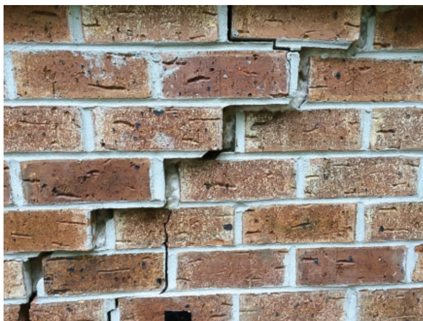
This cracked brickwork is caused by foundation settlement. Photo courtesy Ram Jack.
