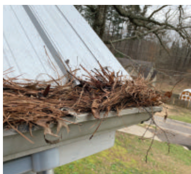
Clogged gutters can lead to rot, insects and foundation problems.
