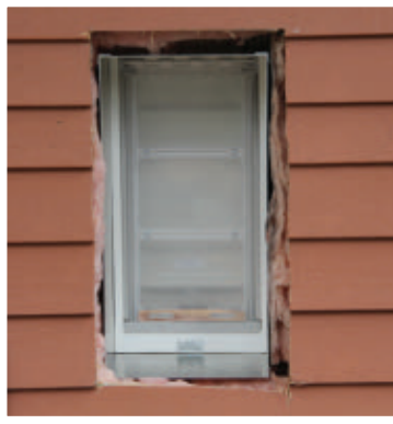
Shown is the wall tunnel with the interior unit in place.
