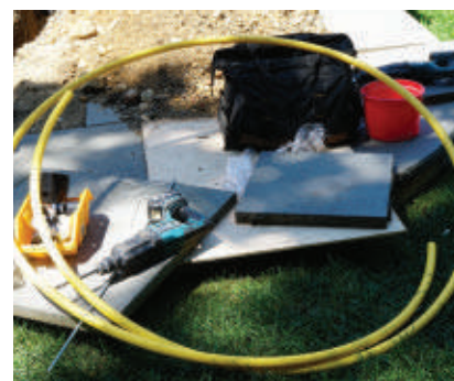
The flexible gas line was installed beneath a patio covered with bluestone tiles.
