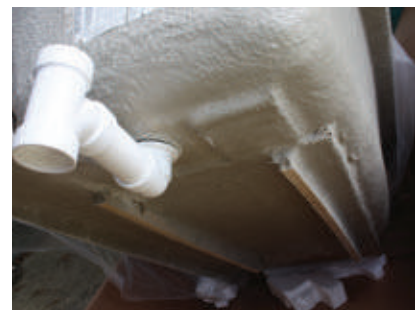
This photo shows the runners on the tub's bottom which sit on the floor. A mortar bed must fill the void between the floor and the tub to support the bottom completely.
