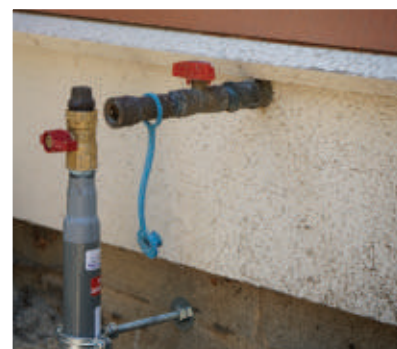
The gas line included a shut-off valve at the house's foundation wall.
