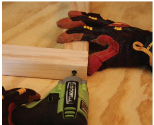
The L-brackets are made of 2x2 material and prevent the sheets from spilling out of the rack.
