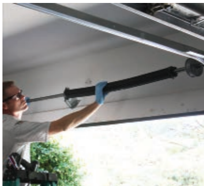
The torsion springs are mounted above the door on a center bracket.
