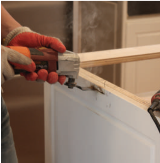
Here an installer notched a cabinet base for a countertop support.
