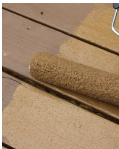
The second coat with the additive is rolled in place. Note the crack on the left side and how it is being filled.
