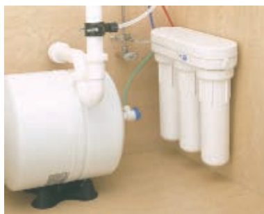
For improved drinking water, we install a point-of-use filter, Pentair RO 3500 reverse osmosis unit.
