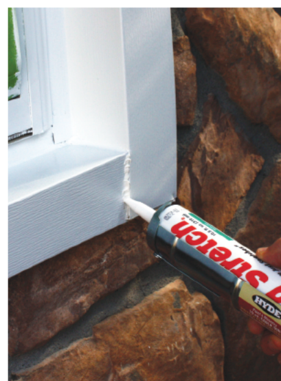
Seal leaks between nonmoving parts (i.e., between door frame and wall) with caulking/sealant.
