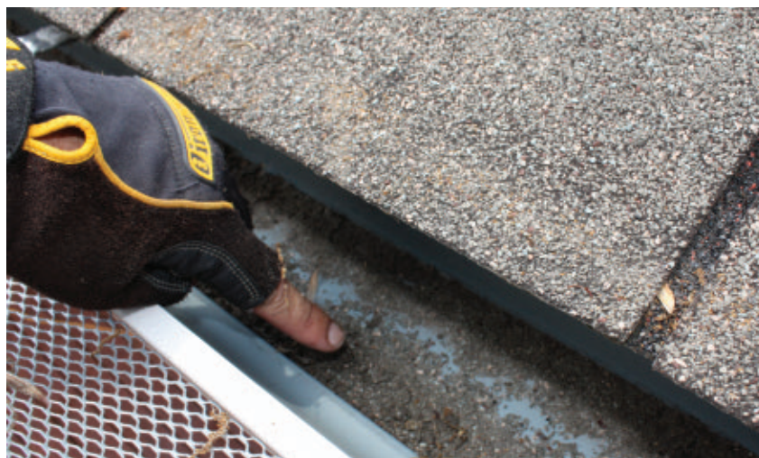
Excessive mineral granules in the gutter can be an indication of wear on asphalt roof shingles.
