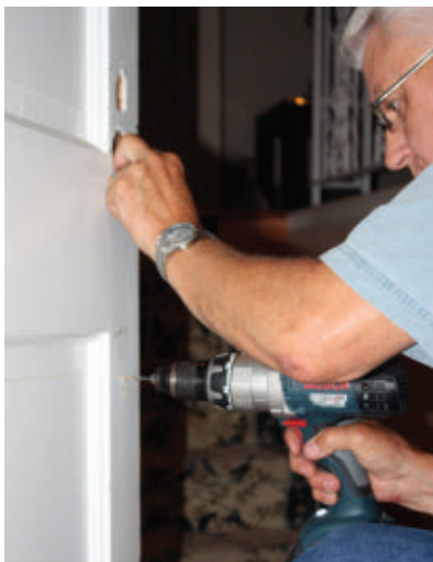
A through-bolt anchors the bottom of the handle to the door.
