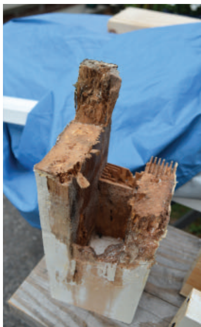
The wood of the post was severely rotted and damaged by ants.
