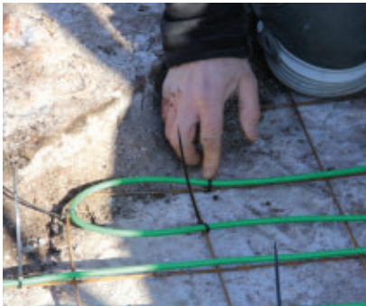
The heating cable loops back and forth in the walkway.
