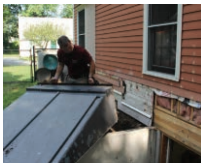
After the old door was removed, the old concrete foundation was found to be in good shape.
