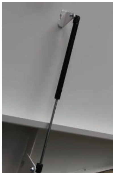
The pistons assist in easily opening and closing the heavy metal doors.
