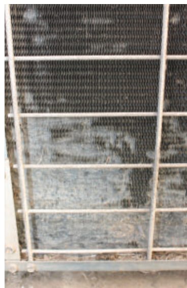
Crushed fins on the side of a condensing unit. Not the end of the world, but it's an avoidable thing that diminishes the performance of the system.
