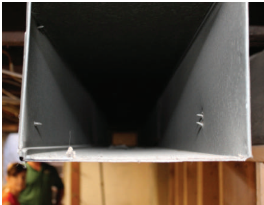
This is a grossly undersized supply trunk. This system never had a chance to operate at peak performance—or anywhere near it.
