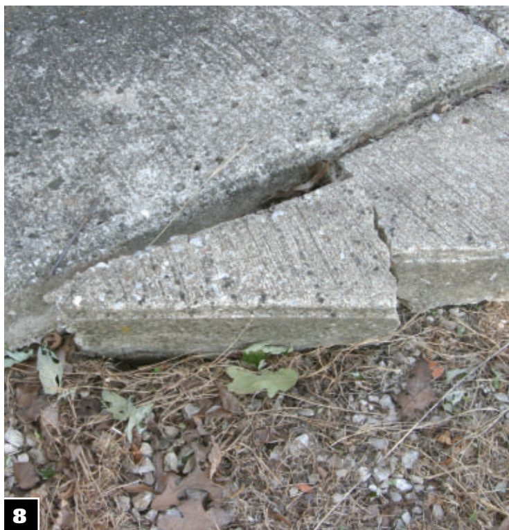
Broken corners and sidewalk slabs require a bit more work.
