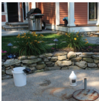
The metal stand of a patio umbrella created unsightly stains on the patio surface.
