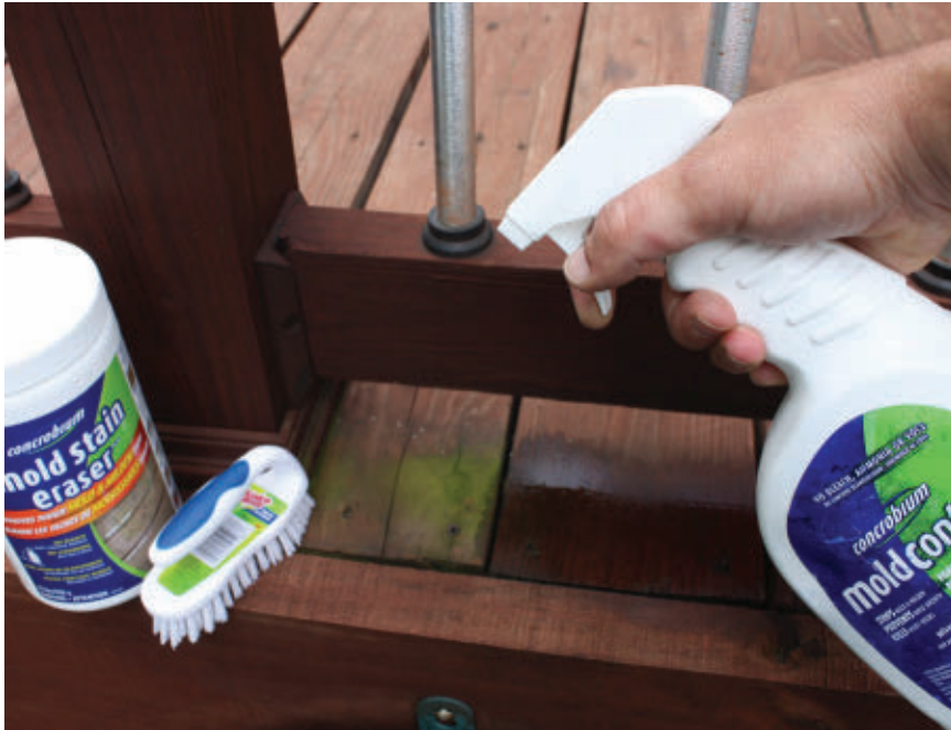
Spot cleaners such as Concrobium Mold Control can be used on targeted applications like the mildew forming on this deck.
