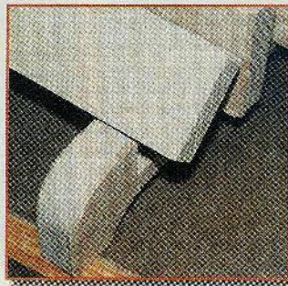
Fig. 12. Use a combination square and a sharp pencil to mark a line 3/4" away from the ends of the cross slats.
