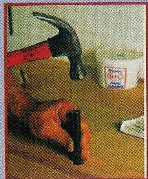
Fig. 3. Using a piece of pipe to hammer a "T" nut into its countersunk hole.
