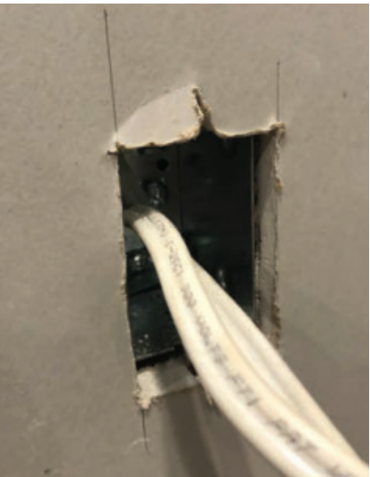
Cut, Don't Rip – This outlet was cut a bit too tight and when the sheet was pressed in place a small piece broke, which in this case isn't the end of the world. Resist the temptation to pull the broken portion off, as it will likely cause the problem to get bigger.
