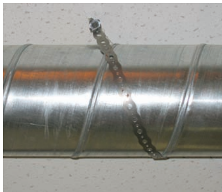
Spiral duct strapped to ceiling
