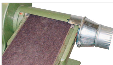
Heating/ventilating pipe reducer, modified and non-riveted into place
