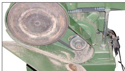
Dust build up below motor pulley
