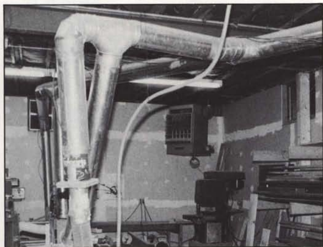
Galvanized tubing connects the blower to the equipment.
