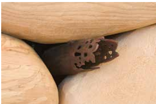
The rusty tailpipe in the wall.
