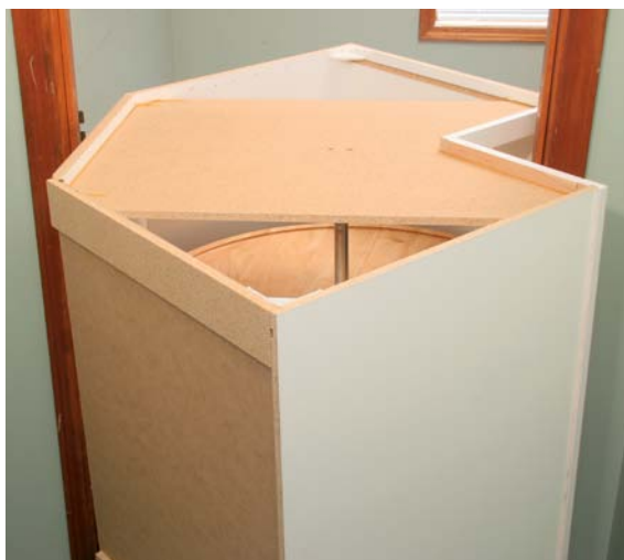
In some cases, getting into the installation room can be a snug situation. Here's a base corner unit that just fit into the laundry room.
