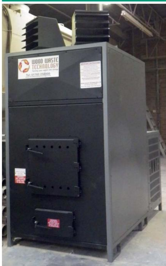
The WT10 wood waste heater installed at Bath Bespoke
