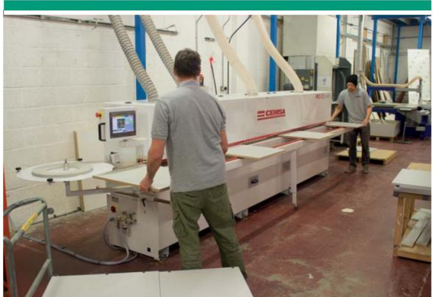
The new CEHISA Pro-12 edgebander installed at Intrafit
