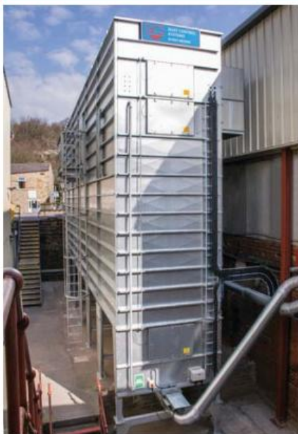
DCS installed two identical Schuko ECOVAR VALIDUS modular filter units, providing JJO with a total extraction capacity of over 190,000m 3 /hr.
