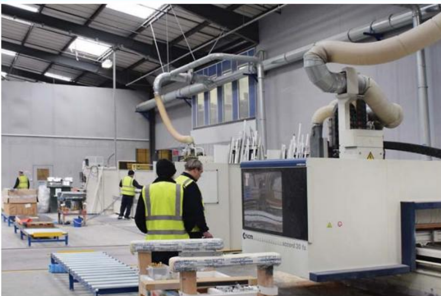
A section of the spacious production area at Distinction Doors – Ecogates dampers are fitted in the main ducting runs.
