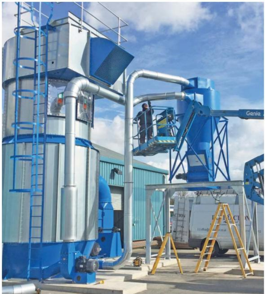
Dustraction's new dust management system at the factory of kitchen and bedroom fitted furniture makers East Coast Fittings.
