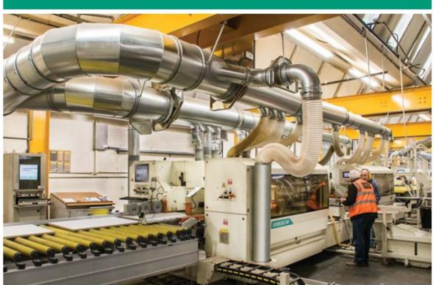
A section of JJO's production line with newly installed ductwork and Ecogate® dampers.
