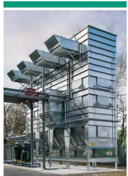
DCS installed a Schuko ECOVAR VALIDUS modular filter unit with 46,850m 3 /hr extraction capacity.
