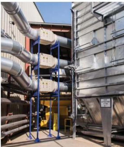
In compliance with ATEX recommendations, the DCS installation includes a total of 10 explosion isolation flap valves.
