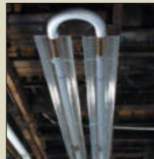
11 Heating and Ventilation
