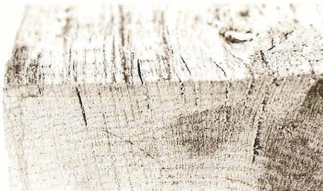
Fig 6.30 Surface checking, following the medullary rays, may not penetrate very deeply; most of this piece is likely to be usable
