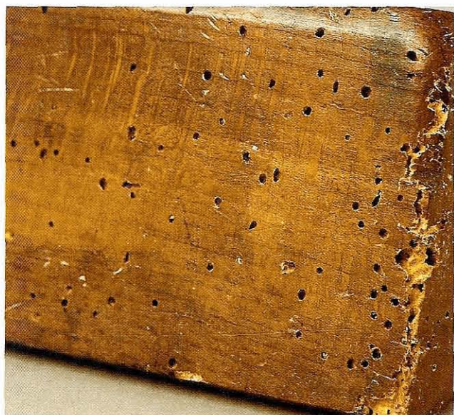
Fig 6.46 Classic woodworm damage: the single surface holes lead to extensive tunnelling beneath. The absence of light-coloured dust suggests that these holes are not recent
